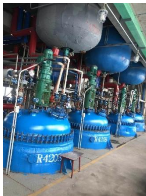
o-Cresol derivatives manufacturing equipment at Wuhai manufacturing plant
