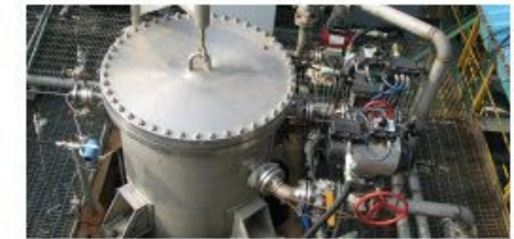
Installed filtration skid system at your site
